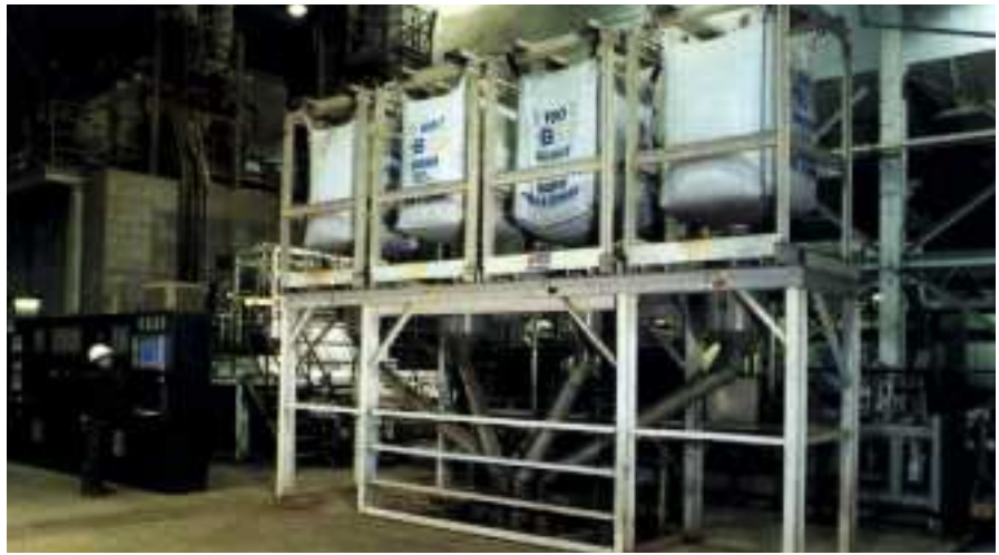
Unilock's Chicago plant has a low-maintenance granular coloring system that runs continuously for nine months a year and produces little dust.
