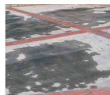
Poor Subgrade Quality
