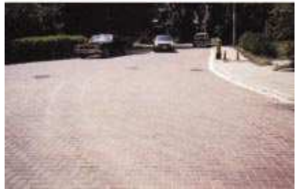
Pine Crescent, a residential brick street in an established, up-market neighborhood in Toronto, Ontario, was removed and replaced with 70,000 s.f. (6,500 m 2 ) of mechanically installed concrete pavers.
