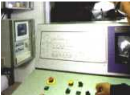
The control panel for the Granumat automated coloring system at Unilock Chicago (background) is linked to the plant's control system.
