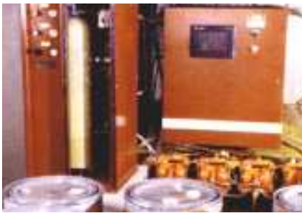
This liquid coloring system was recently installed at A-Block, a CMU producer in Needles, Calif. Liquid colors are drawn out of drums through a hose or pipe that set on top of the drums. Four pumps (center of picture) are used, one for each of the basic iron oxide colors. The cylinder in left cabinet rests on a load cell to meter the amount of liquid colors programmed into the control panel on right. Colors are then transported to the concrete mixer.
