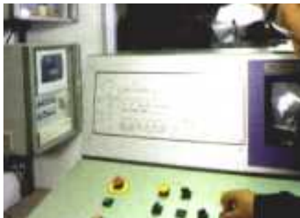
The control panel for the Granumat automated coloring system at Unilock Chicago (background) is linked to the plant's control system.
