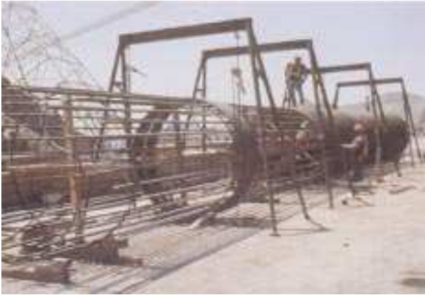
Front end of the parking structure is founded on huge concrete caissons sunk to depths of 90 ft. Here workers assemble a steel cage for one of them.
